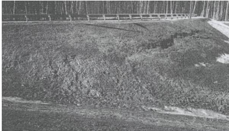
Figure 2. Local deformations of subgrade embankment:
